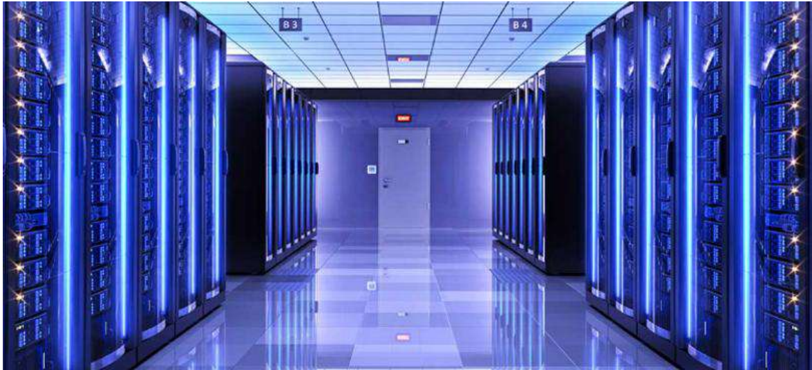
Data Centre Infrastructure Solutions
